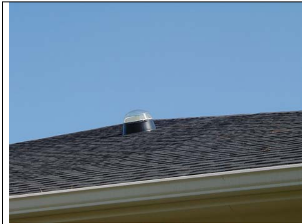
Solatube on roof
