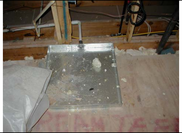
Rinnai sealed combustion through roof
