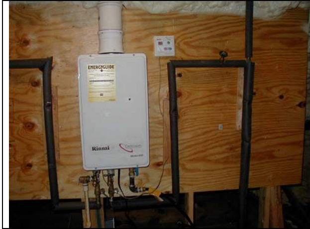
Rinnai Continuum Instant Hot Water in Attic
